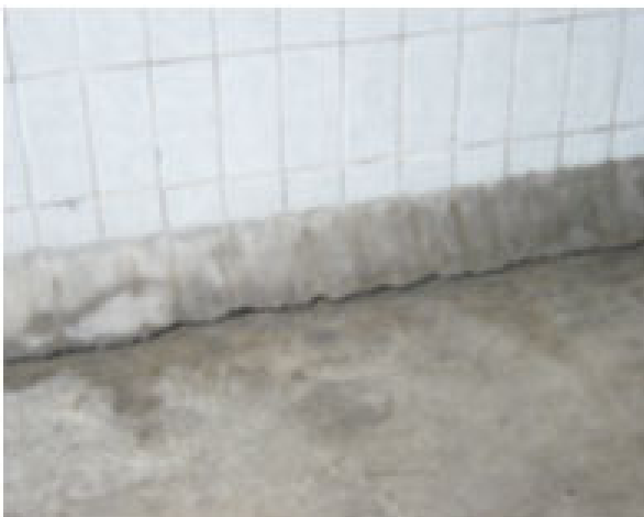
Fig. 474: Proper cleaning/sanitation not possible. Crack in junction wall/floor
