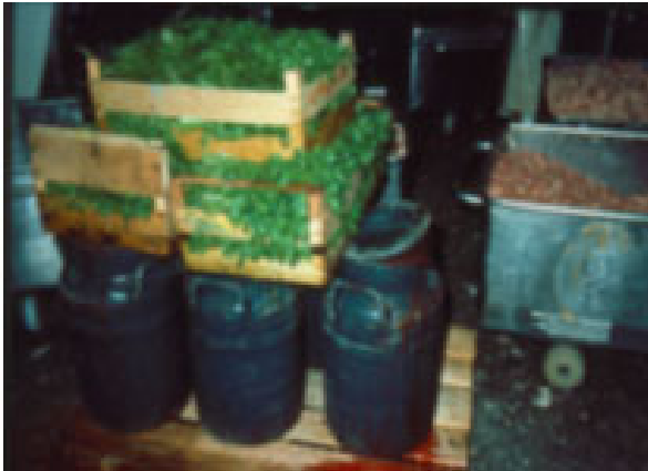
Fig. 476: Minced meat and vegetable in same chiller - risk of cross-contamination
